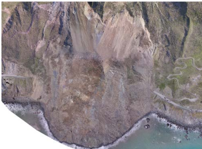
Above: Aerial photo of Mud Creek on May 25, 2017.
